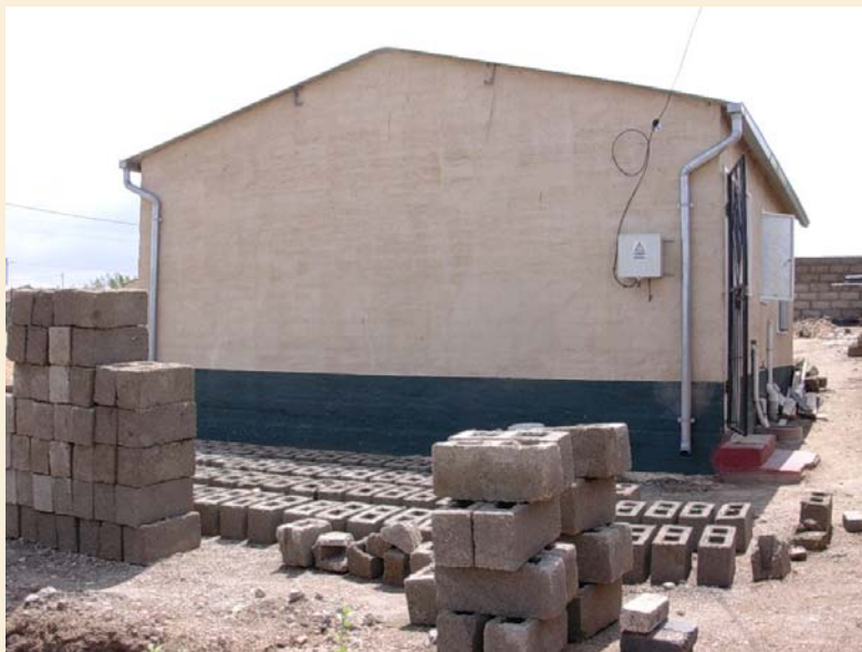
Acquiring the materials to build a wall around a bonded house in Diepsloot, South Africa
